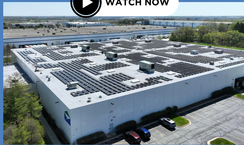
One of Illinois's Largest Rooftop Solar Projects
